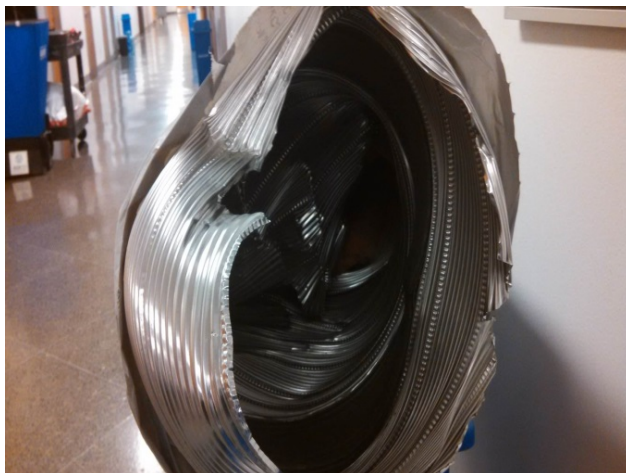
Aging HVAC Systems (Damaged Duct)
